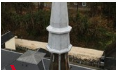
1 Fixing the base and the tapered section to the bell tower gable.
